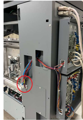
Upstream Finisher Wiring
